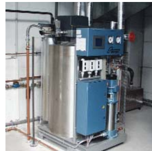
Fig. 7: Heating steam generator
