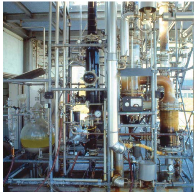
Fig. 1: Acetic-acid recovery unit
