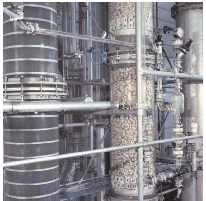
Fig. 1: Sieve plate extraction column and distillation column DN450
